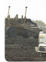
McAninch Corp. is using Trimble Construction Manager GPS hardware and software to closely monitor its fleet of mobile assets.
